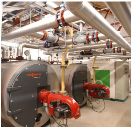
This CHP plant room in Stockethill, Aberdeen supplies heat and power to nearly 300 flats. Image courtesy of Aberdeen City Council
