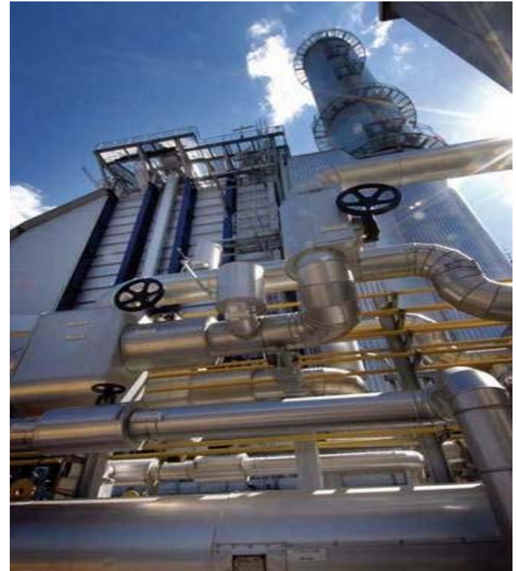
BASF CHP unit 90% fuel efficiency
