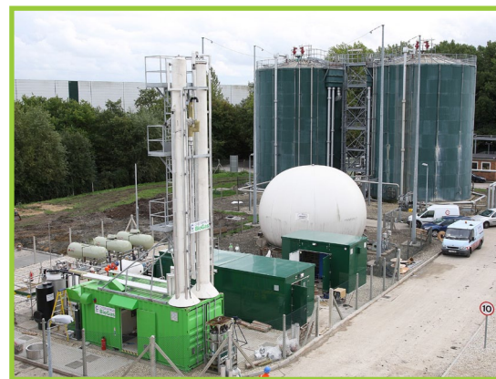
Complete - Gas being put to good use
