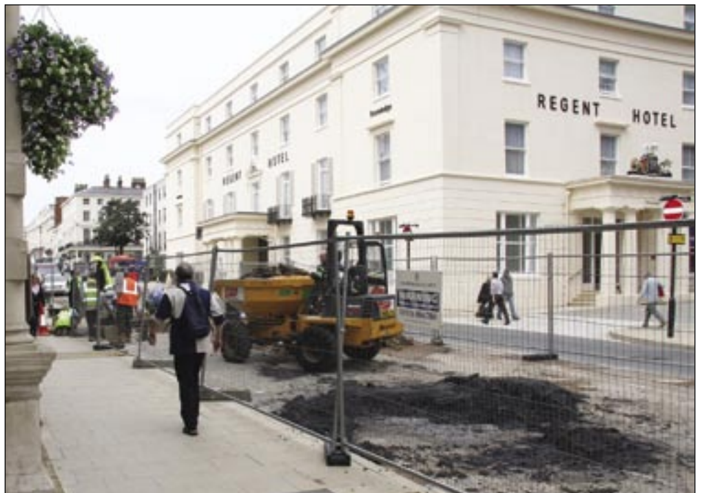
Work in progress on the Parade. Visit www.warwickshire.gov.uk/parade for the latest information.
